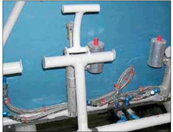
There are several variation of flex lines including the armored Aeroquip lines that make a very neat, compact installation.
