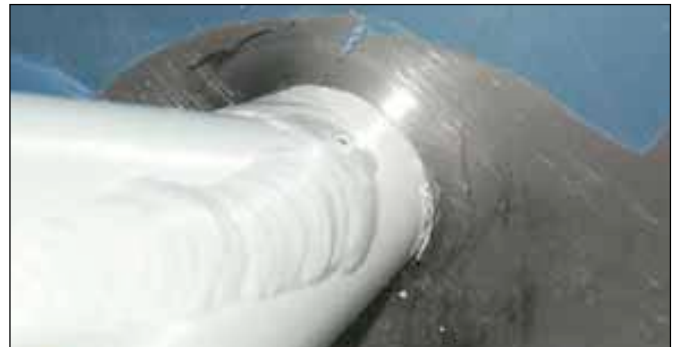
Done carefully, there is little or no gap. If there is a gap fill it with high temperature RTV.
