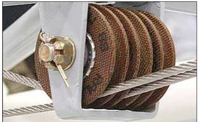
Belly control pulleys looking AFT. The far pulley, left, when looking forward is the cable from the top of the elevator bell crank. The cable from the bottom goes through the middle and the flap cable goes through the right one.
