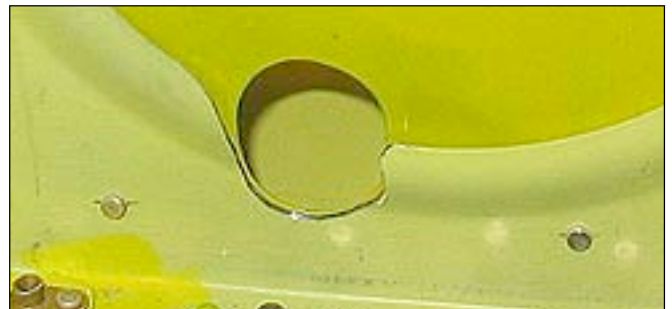
This builder came straight out of his tank, which required a notch in the stiffening bead. This is a no-no unless you go to the additional effort of fabricating a doubler for the area (.025), as he did.
