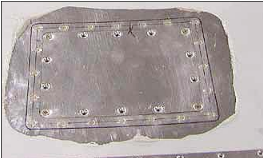
The outside marker line shows the underlying frame outline and the inner one establishes the line for the attaching rivets.
