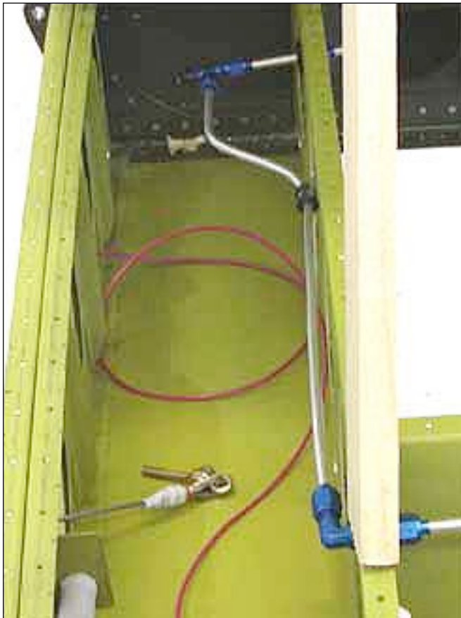
Inboard bay, looking forward, right wing. An AN ninety-degree bulkhead fitting is used to make the corner and an AN "T" fitting put in the top sight gauge line.
