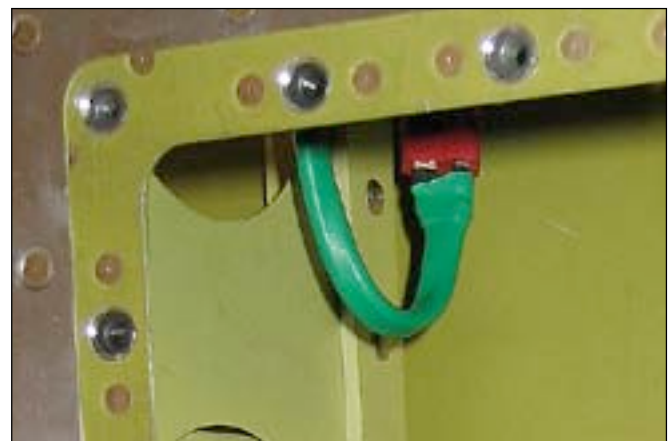
When countersinking for tank or general access covers, try to cut the minimum needed so you barely touch the nut plate.
