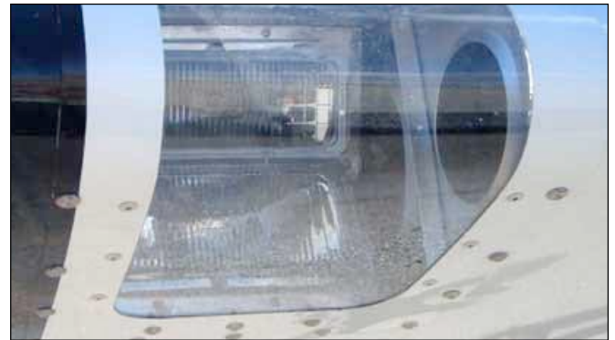
To mount it in the wing, a .032 doubler must be riveted around the cut out. The lights used here are auto high beams.
