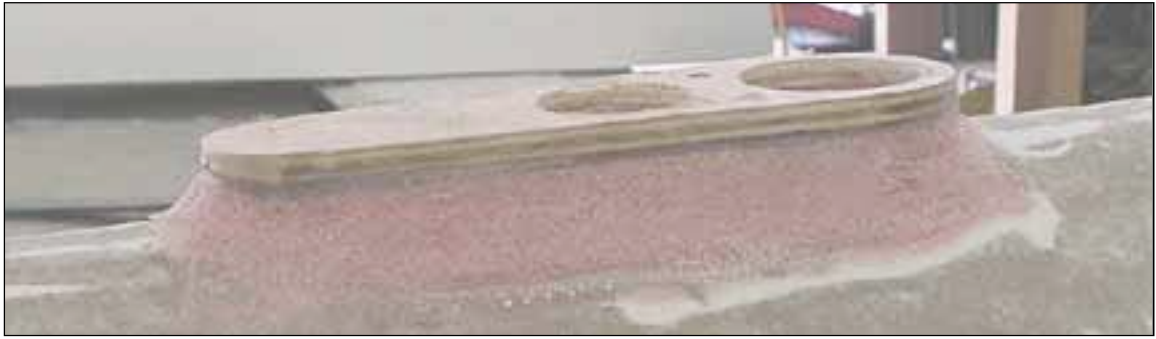
Strobes/nav lights need a solid base to attach to. This builder epoxies and fiberglassed a plywood mount in place and faired it in with foam and microballoons. Don't use Bondo, as it is really heavy.
